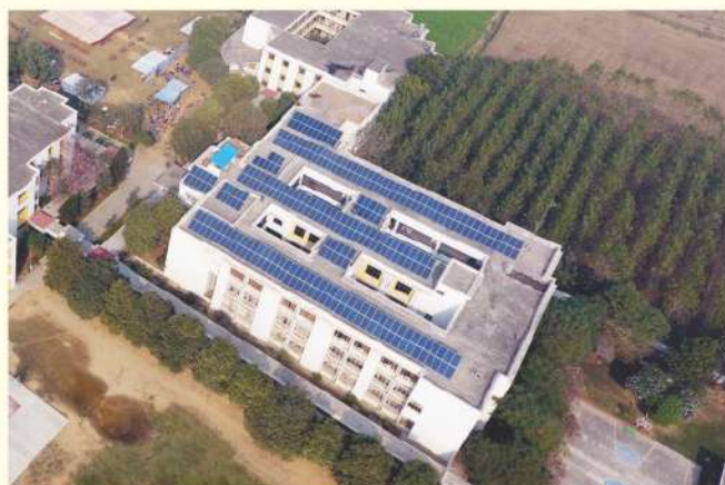
Energy-Saved-Solar Plant - 55 KW
